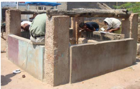
Revival of old unused well for decentralized piped supply for a slum
